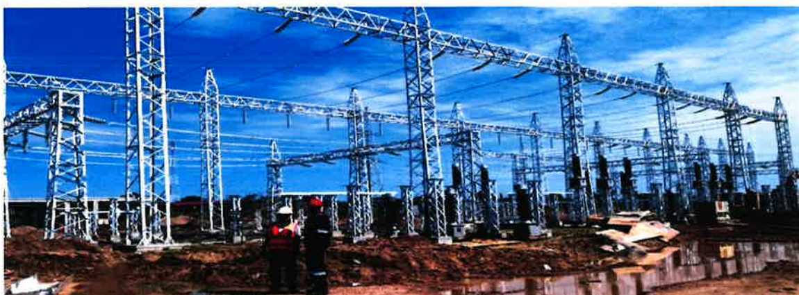
Figure 4 : Switchyard installations at Isimba
