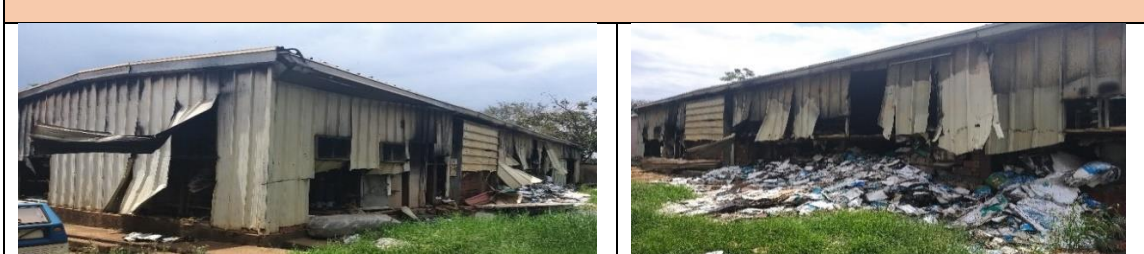
A Section of burnt down stores yet to be restored. The structure discharges hazardous chemical wastes
