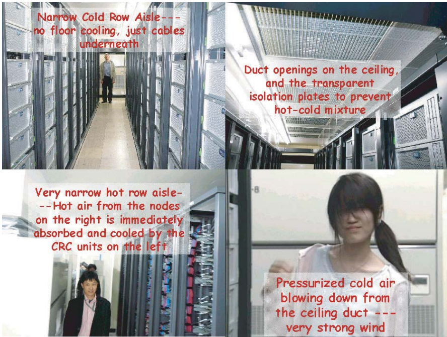
FIGURE 14.6: TSUBAME cooling and airflow photographs — the woman’s hair is blown vigorously with very strong pressurized cooling air from the ceiling plenum above.
